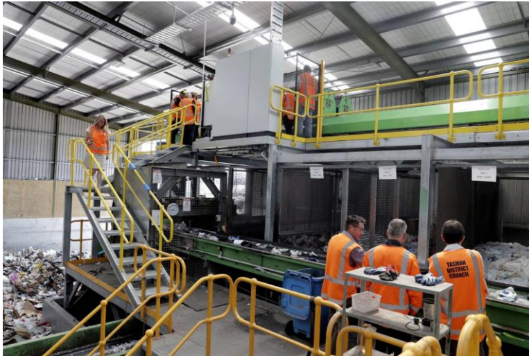
Figure 1: Optical sorting machine installed in the Nelson-Tasman Material Recycling Facility
